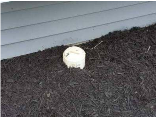
Photo 4-1 Soil in contact with siding.
