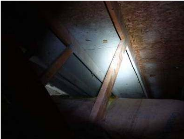
Photo 9-1 Evidence of repair; may be treatment for organic growth.
