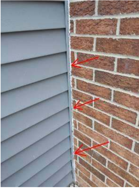
Photo 5-1 Caulking degraded; need to be re-caulked.
