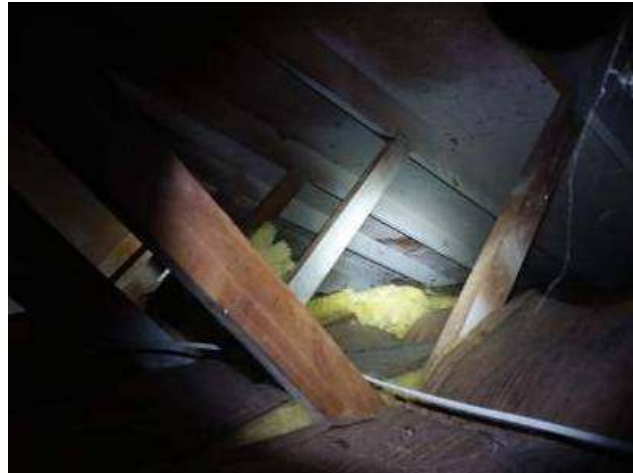
Photo 9-2 Evidence of repair; may be treatment for organic growth.
