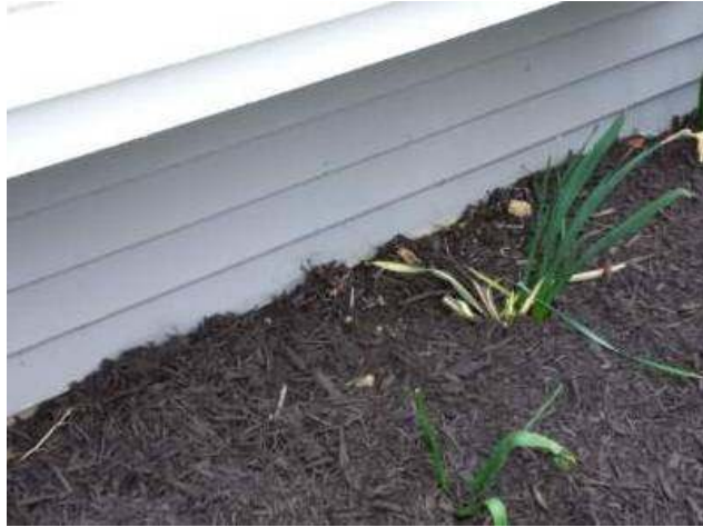
Photo 4-2 Soil in contact with siding.
