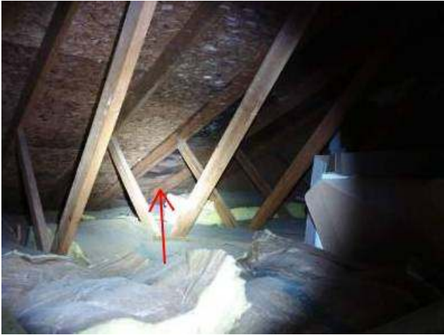
Photo 8-1 Evidence of previous water leak.
