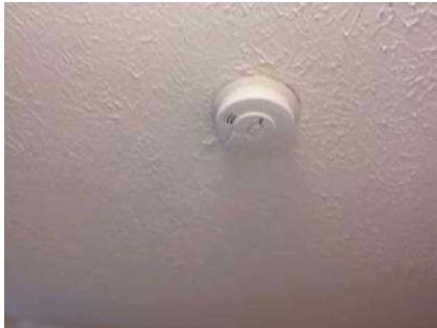
Photo 11-2 2nd floor hardwired smoke detector.
