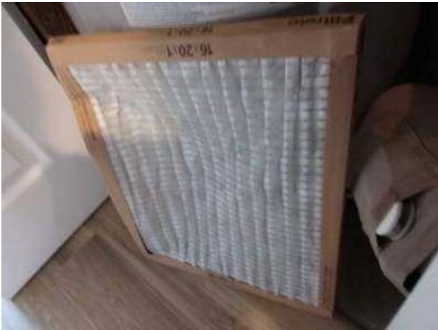
Photo 19-1 New filter ruined during install/removal. No clearance to filter slot resulting from installation of water heater too close to air handler.
