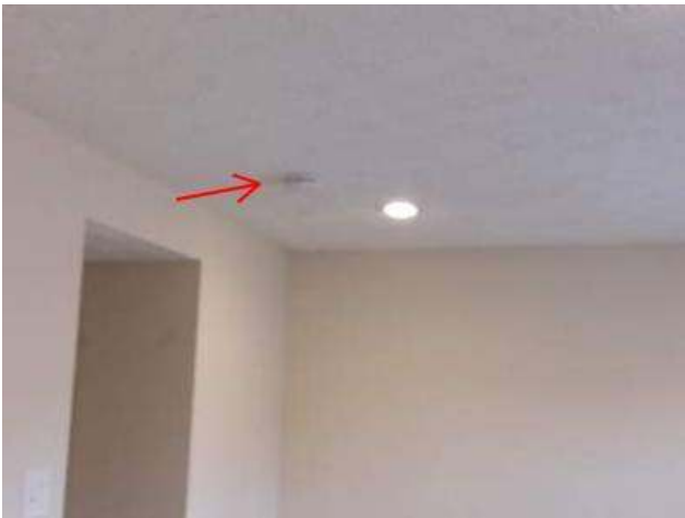
Photo 11-1 1st floor 10-year sealed battery non-hardwired smoke detector.
