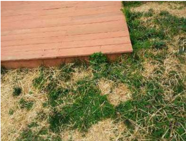
Photo 2-1 Soil in contact with decking structure.
