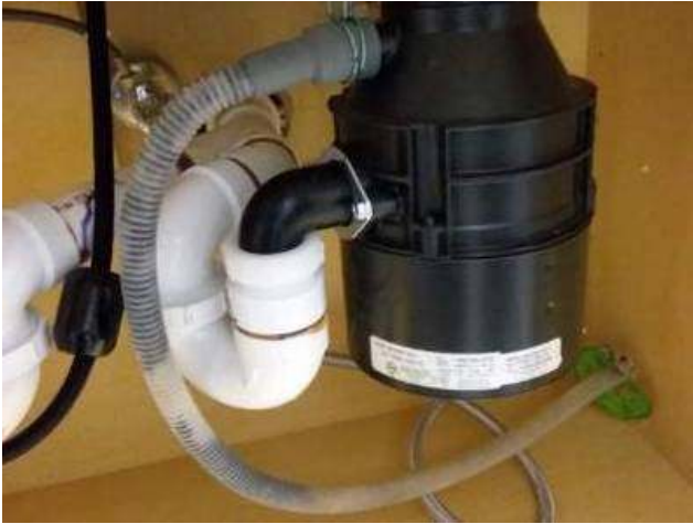
Photo 25-1 No evidence of high loop for dishwasher.
