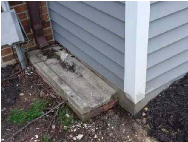
Photo 6-1 Need to extend downspout drain.
