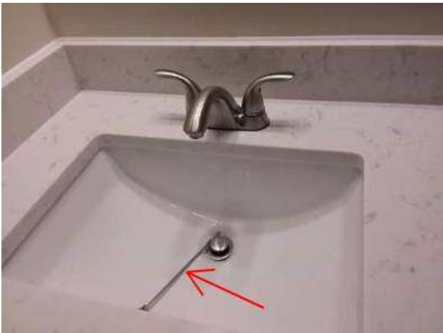
Photo 29-1 Sink stopper not connected.
