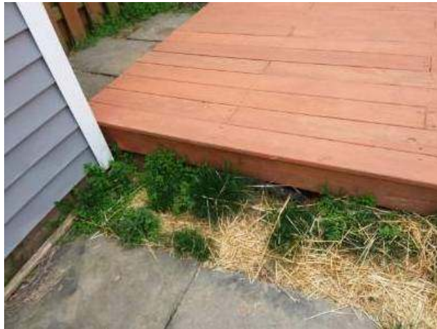
Photo 2-2 Soil in contact with decking structure.
