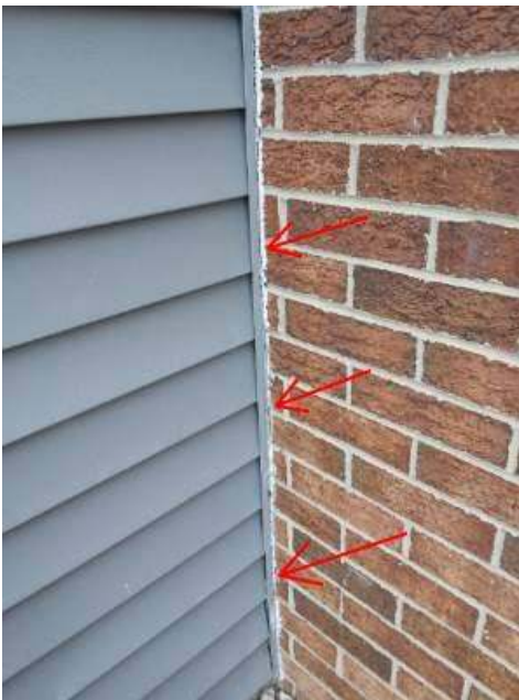
Photo 5-1 Caulking degraded; need to be re-caulked.
