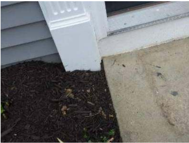
Photo 4-3 Soil in contact with trim.
