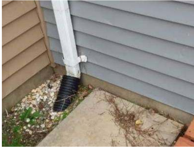
Photo 6-2 Buried downspout line-destination unknown.
