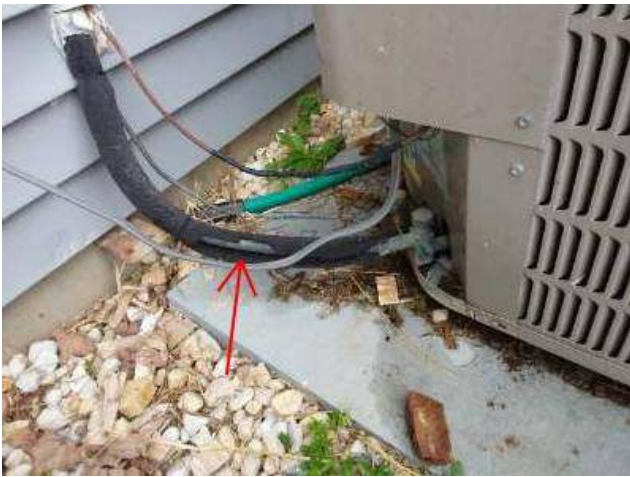
Photo 18-1 Degraded HVAC line insulation needs replacing.
