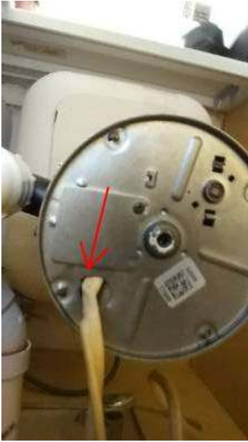
Photo 23-1 Missing wire clamp.
