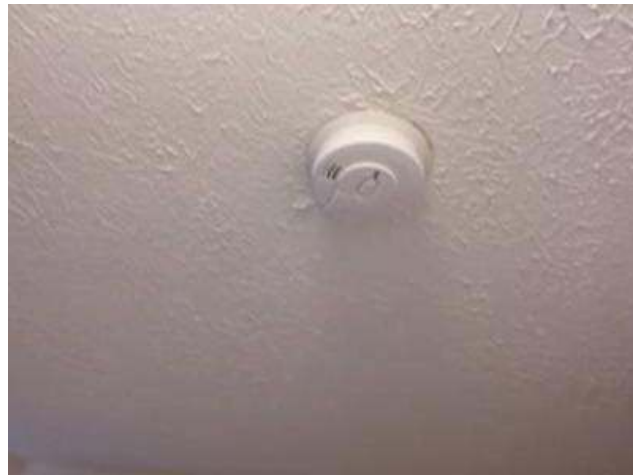
Photo 11-2 2nd floor hardwired smoke detector.
