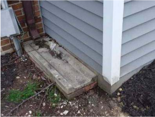
Photo 6-1 Need to extend downspout drain.
