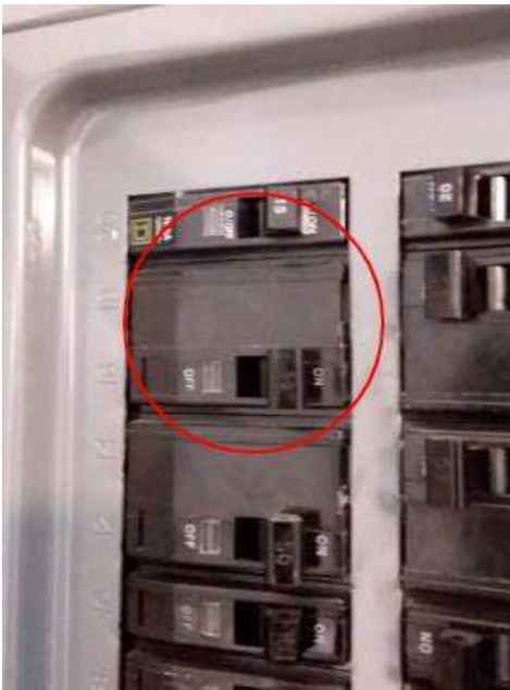
Photo 12-1 30 AMP breaker for HVAC compressor. Compressor rated for 20 AMP.
