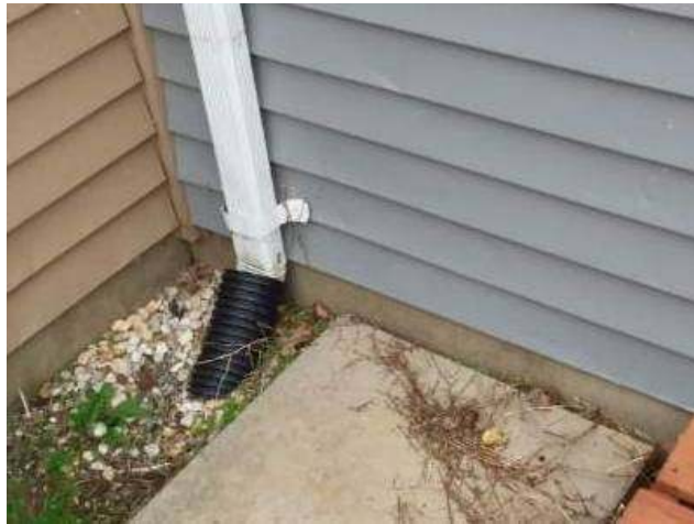
Photo 6-2 Buried downspout line-destination unknown.
