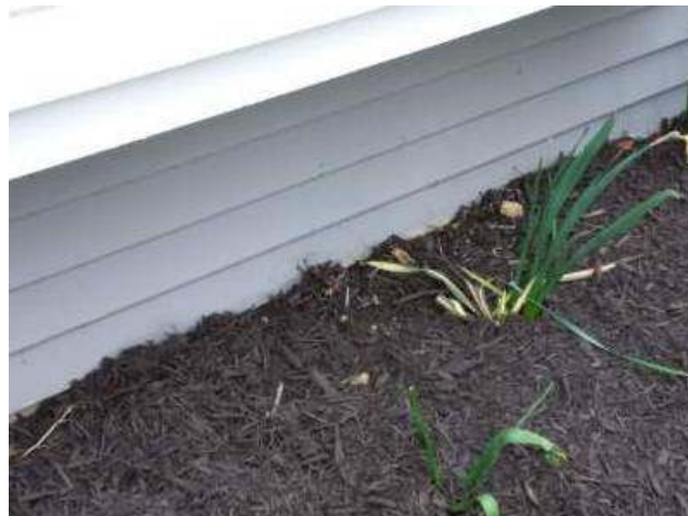
Photo 4-2 Soil in contact with siding.
