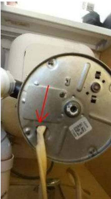
Photo 23-1 Missing wire clamp.
