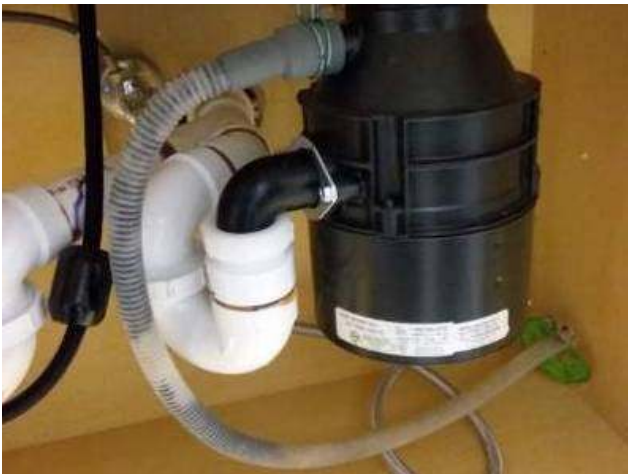
Photo 25-1 No evidence of high loop for dishwasher.
