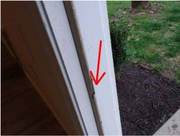
Photo 30-1 Damaged weather seal; needs replacement.
