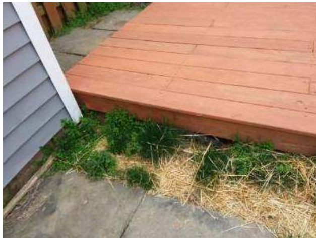
Photo 2-2 Soil in contact with decking structure.
