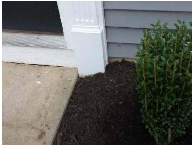
Photo 4-4 Soil in contact with trim.
