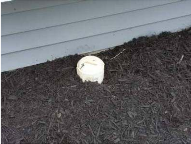
Photo 4-1 Soil in contact with siding.
