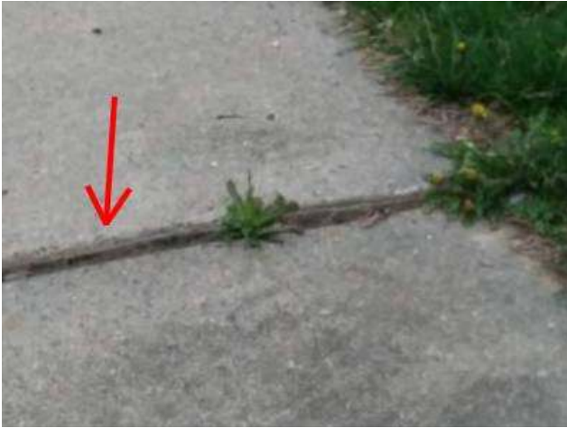
Photo 3-1 Trip hazard on common area sidewalk.
